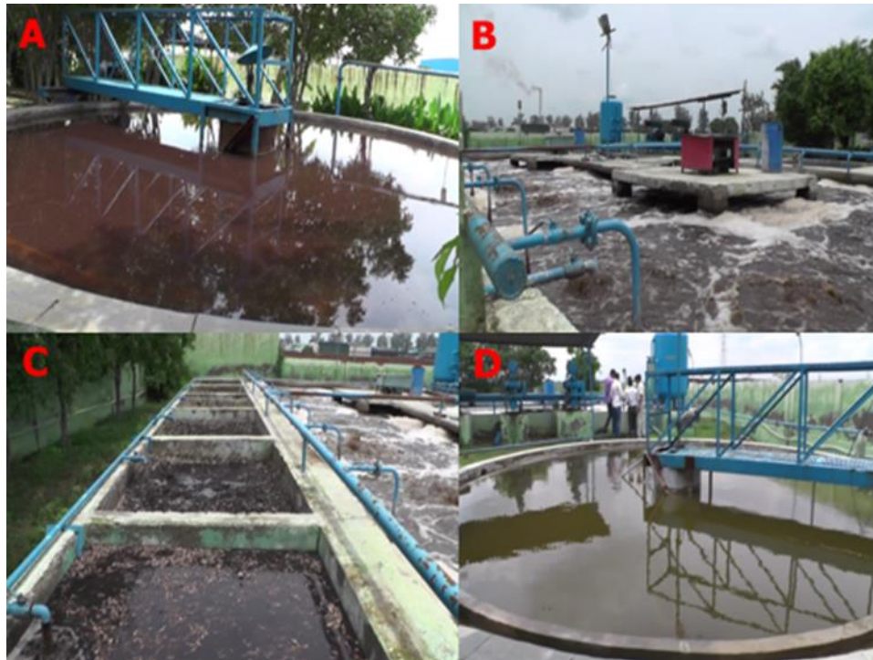
Figure 4: A. Primary clearance tank; B. Ariation tank; C. Sludge activate tank and D. Secondary clearance/ policing tank and Carbon filter.
